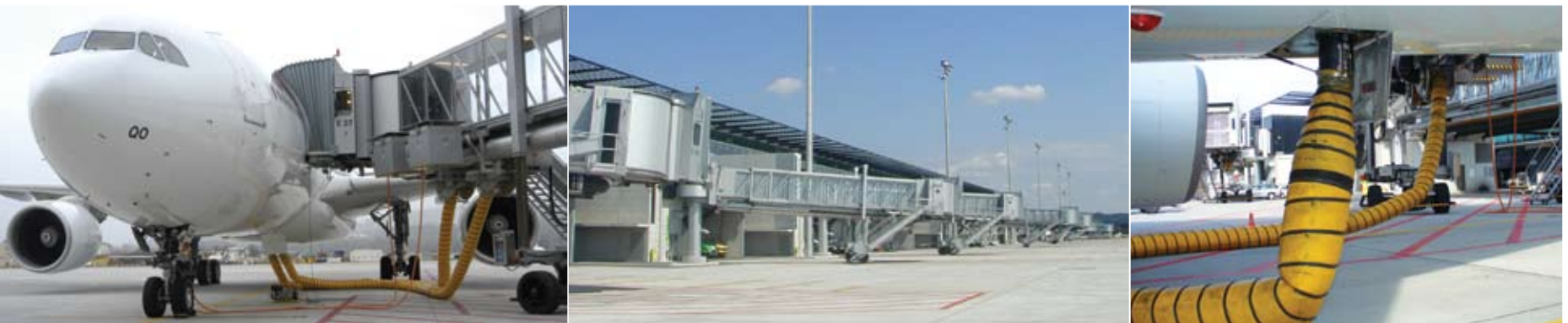
Fixed electrical ground power and air conditioning
