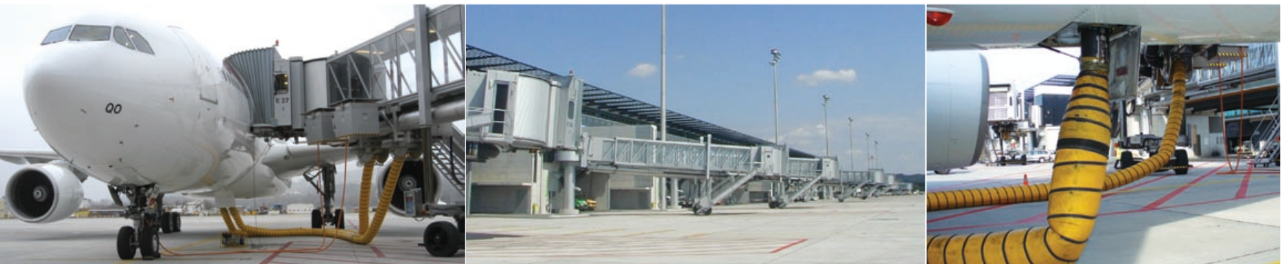
Fixed electrical ground power and air conditioning
